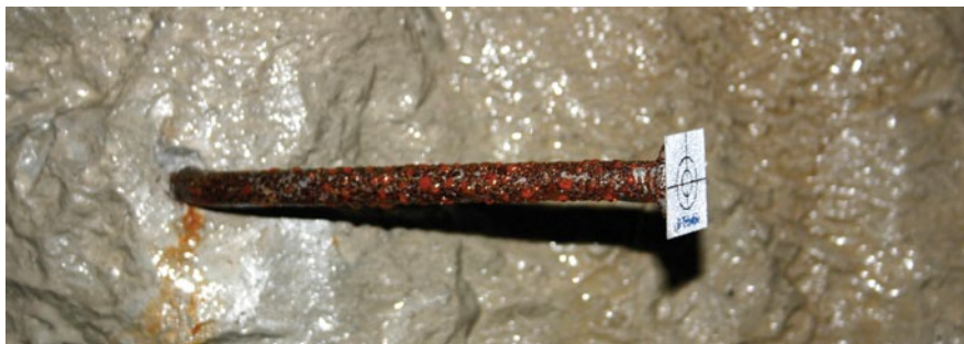
Spike set in wall with epoxy glue and adhesive target used for control. This method was later replaced with threaded bolts and spin- on prisms.
