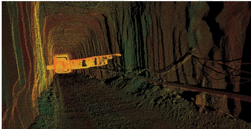
Point Cloud of decline and bench area in background created with Trimble GX 3D Scanner and Trimble RealWorks Survey software.
