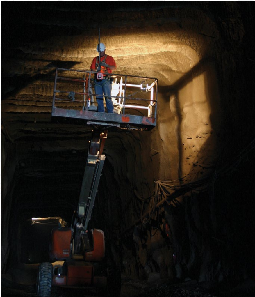
Grant Van Bortel, V3 Technology Manager, aboard a manlift, using an inverted prism pole staking out bolt locations on the ceiling of the decline in preparation for the conveyor installation.
